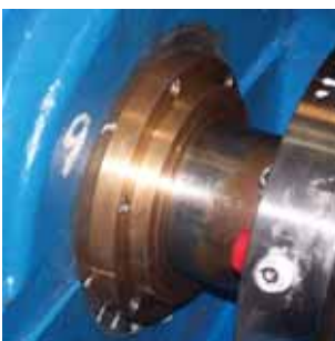
Flange mounted LabTecta-RDS™ installed on a double ended pump (Case Ref: 3304)
